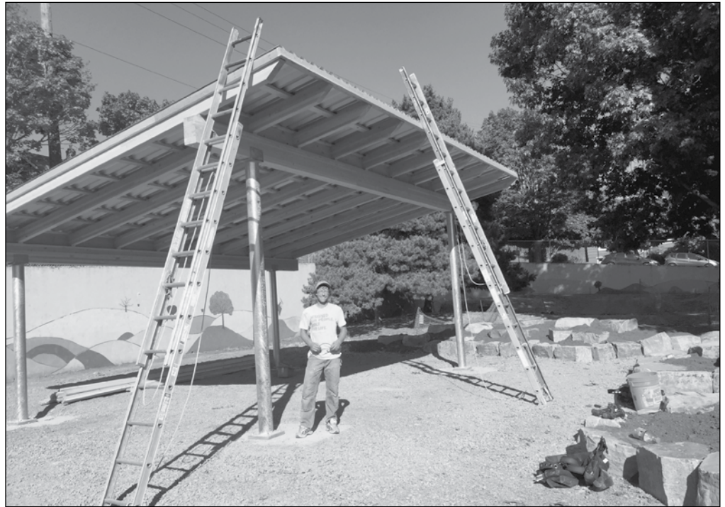
A worker from Green Hammer Construction stands under the new outdoor classroom under construction.
